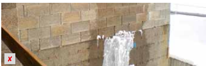
Vlažni tzv. mantelbeton
